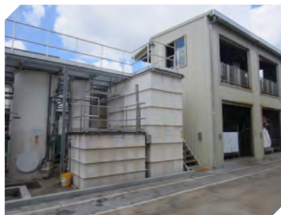
San Shing's mixed wastewater treatment plant
